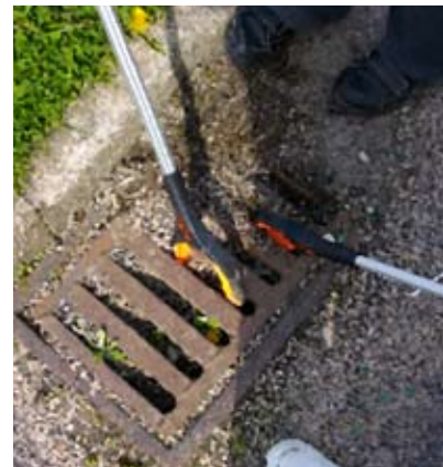
We reported blocked drains so that they could be fixed.
